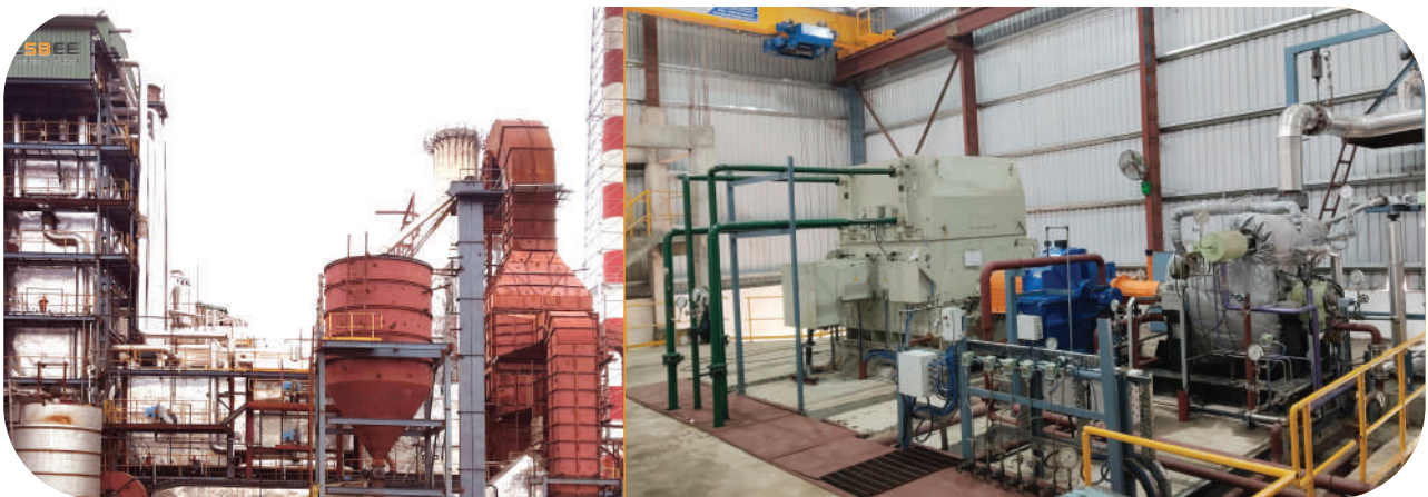
IPP Power Plant
