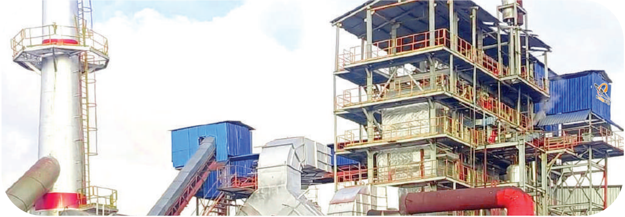
COGEN Power Plant
